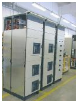
Megalopolis Power Plant
