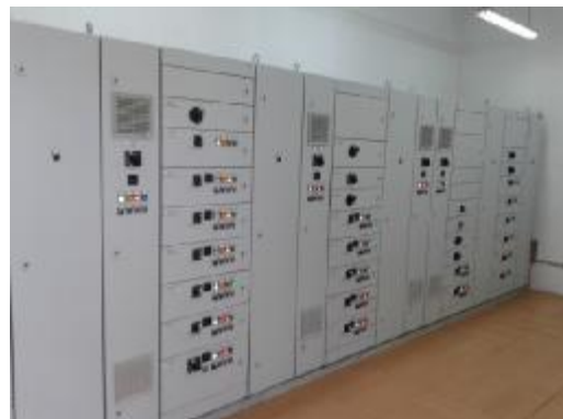
Baia Mare waste water treatment plant
