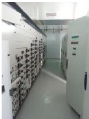
Tan Tan water treatment plant
