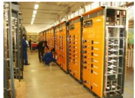
Lichtenburg Cement Plant
