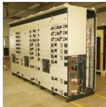
Craiova Power Plant
